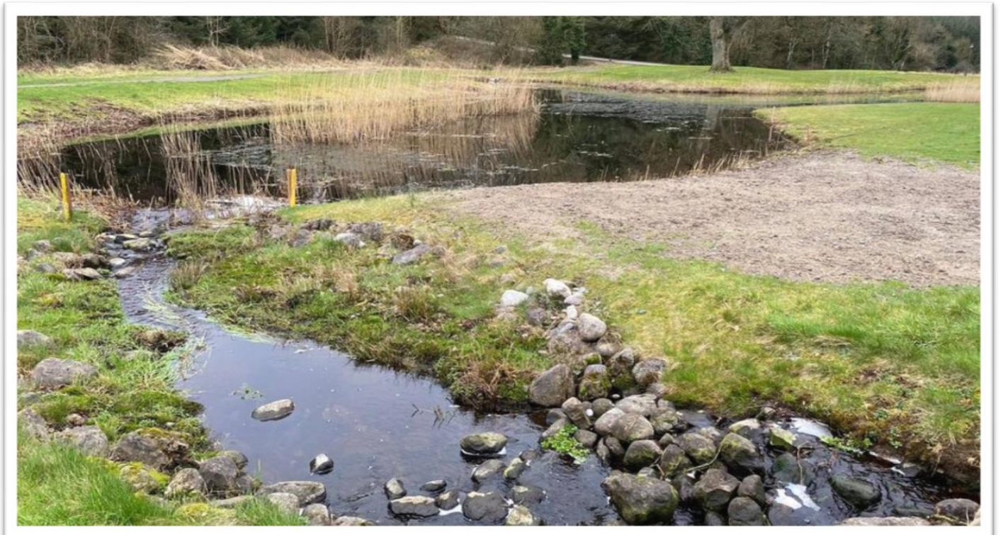
The stream and lake on the right of the 5 th hole have also been cleared
